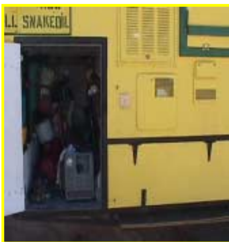
Generator & storage compartment. Also shown are vents for refrigerator, furnace, and water heater
