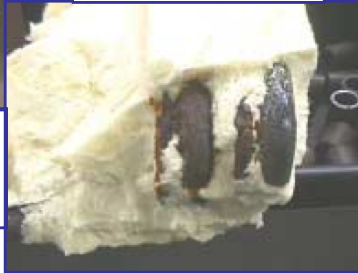
Below: Close-up view of damaged evaporator. Note extensive rust damage.
