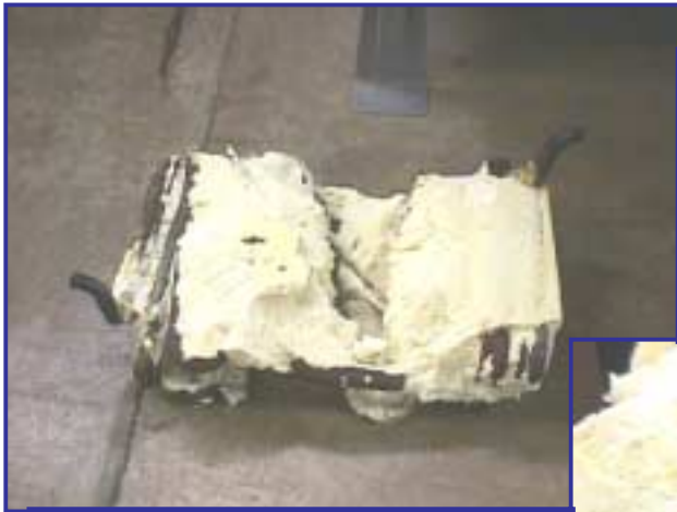
Above: Deteriorated evaporator.
